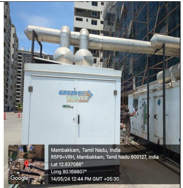
DG Set of 500 KVA Capacity – 2 Nos for commercial building.
